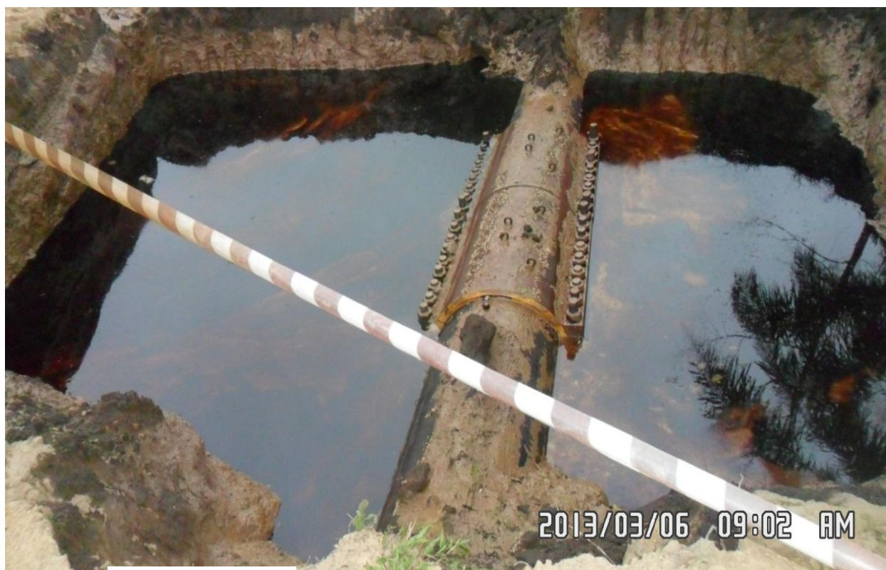
Figure 1: Faulty pipeline along the SPDC Right of way at Rumuolukwu
